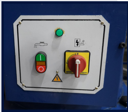
POWER CONTROL PANEL
