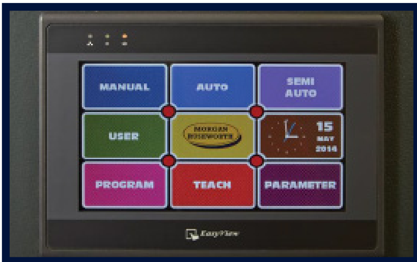
NC CONTROL PANEL SCREEN
